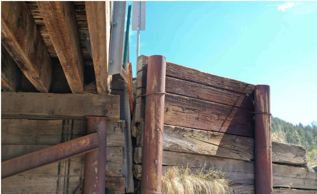
Picture 3 – Wingwall Separation
